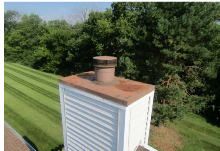
rust at cover
