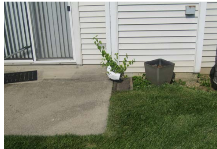
downspout discharges too close to building
