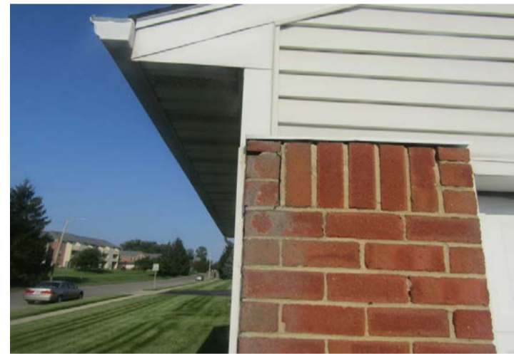
isolated mortar deterioration
