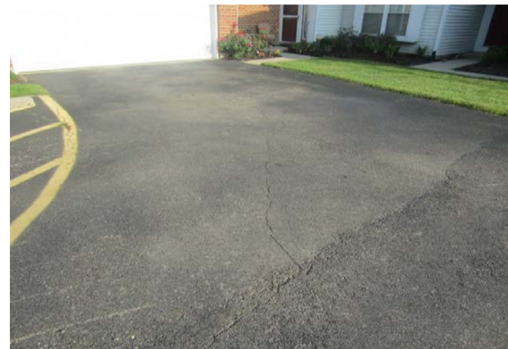
crack in pavement
