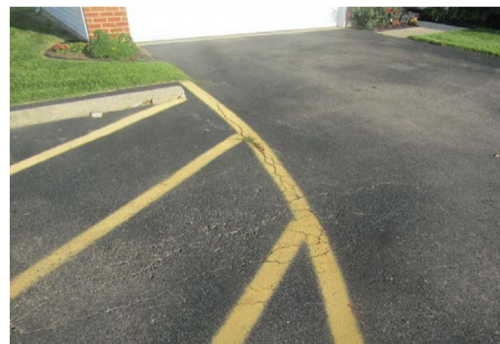
cracks in pavement
