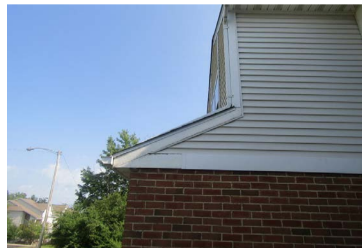
missing cladding at 2332 Raider
