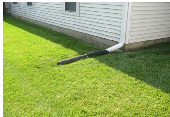
surface extensions are unsightly and prone to damage
