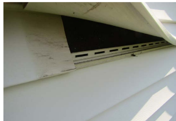
missing building paper
