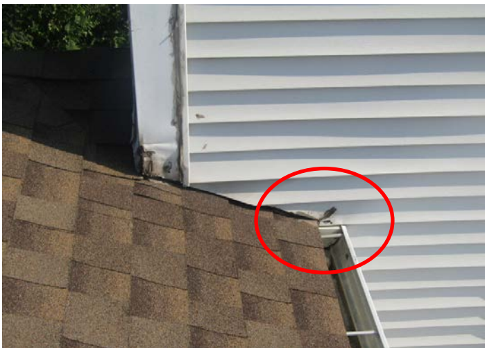
missing kick-out flashing and reports of leaks at 1473 Eagle Highlands
