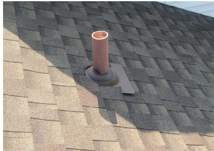
loose flashing requires securing - address with semiannual inspections
