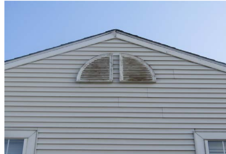
finish deterioration at decorative gable vents
