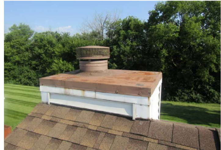
rust at cover
