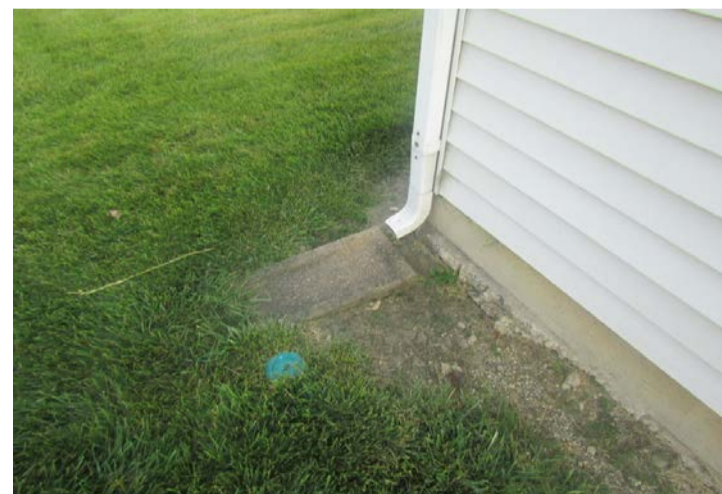
downspout discharges too close to foundation (splash block not installed properly)
