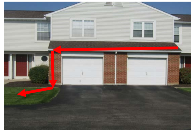
reroute gutters and downspouts at garages to discharge into adjacent grass
