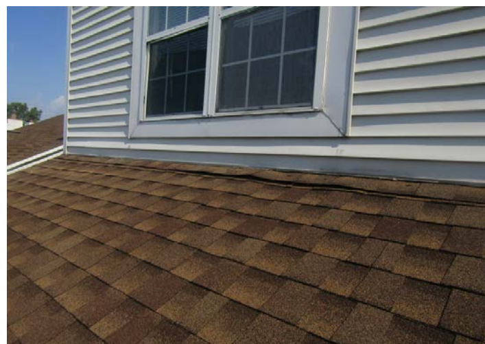
upper shingle course at roof to wall intersection requires securing
