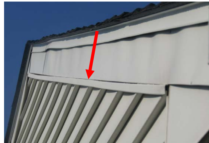
water can get between fascia and J channel if caulk fails
