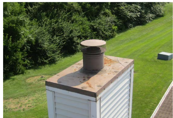
caulked cover at 1473 Eagle Highlands - leaks at chimney
