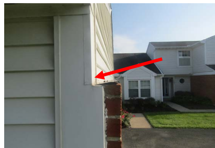
flashing is pitched towards the building increasing the potential for leaks
