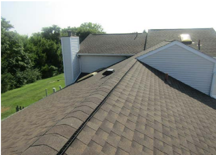
ridge vent with wind baffles
