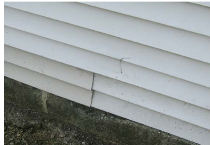
damaged and unmatched replacement piece
