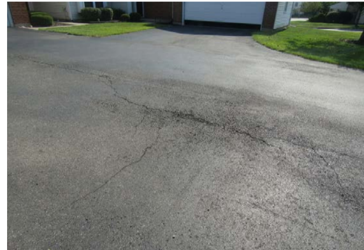
raveling (loss of surface material)
