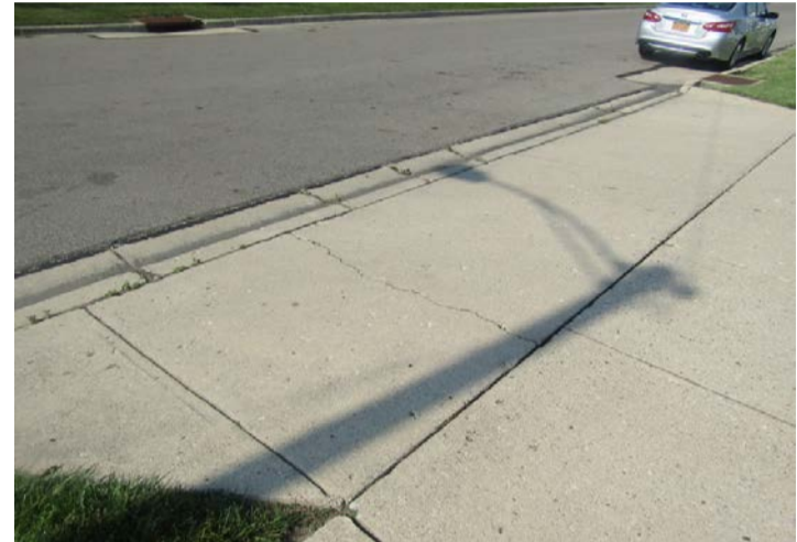
cracks in concrete
